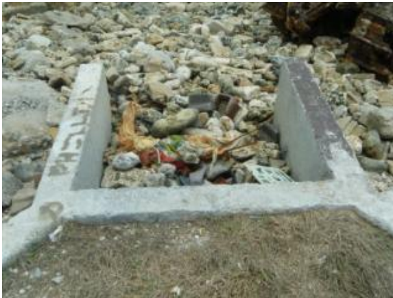
Figure 2.20 - Outlet headwall filled with debris
