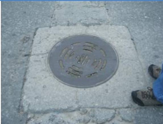
Figure 2.14 - Dirt can be seen up to the cover of this drywell
