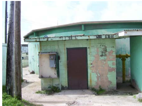
Figure 3.12 – FW Booster Pump House Central (typical)
