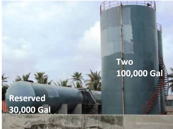
Figure 4.3 - Diesel Storage Tanks
