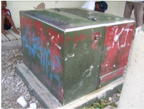
Figure 4.23 – Typical pad-mounted transformer
