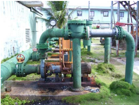
Figure 3.6 - Well Pump 1 (South)
