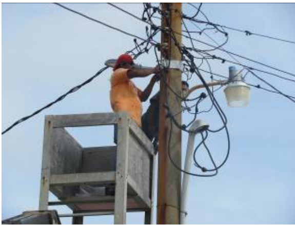
Figure 4.9 – Upgrade Street Light to LED Fixture
