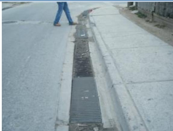
Figure 2.16 - Dirt can be seen up to the top of the grill on these trench drains
