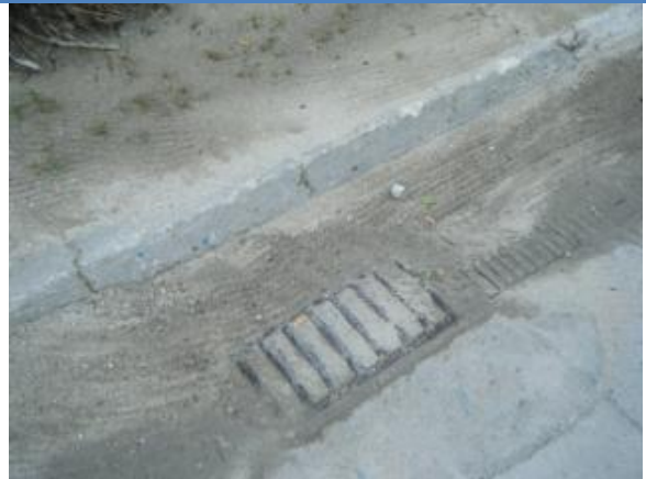
Figure 2.15 - This side drain is filled with sand
