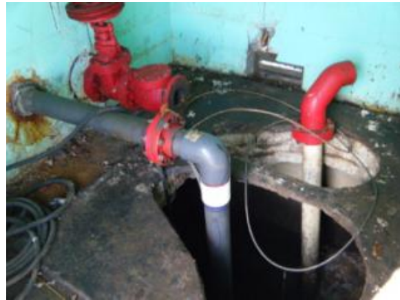
Figure 2.11 – Lift station #2 original pump and backup are no longer there
