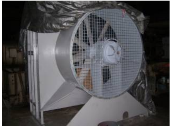
Figure 4.28 – Replace Leaking Radiator on Generator #3
