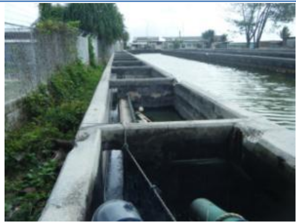
Figure 2.3 - V-notch weir and effluent box
