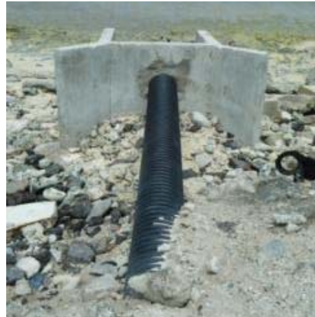
Figure 2.21 - Outfall exposed due to erosion
