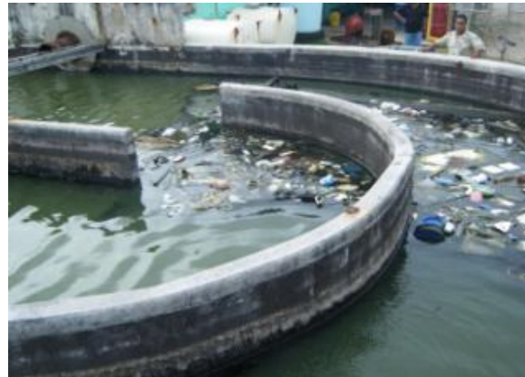
Figure 2.5-Debris and rainwater in the oxidation ditch
