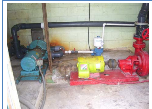
Figure 3.13 – FW Booster Pumps
