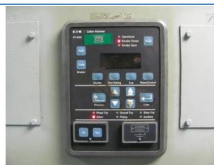
Figure 4.8 - Typical Feeder Relay Panel
