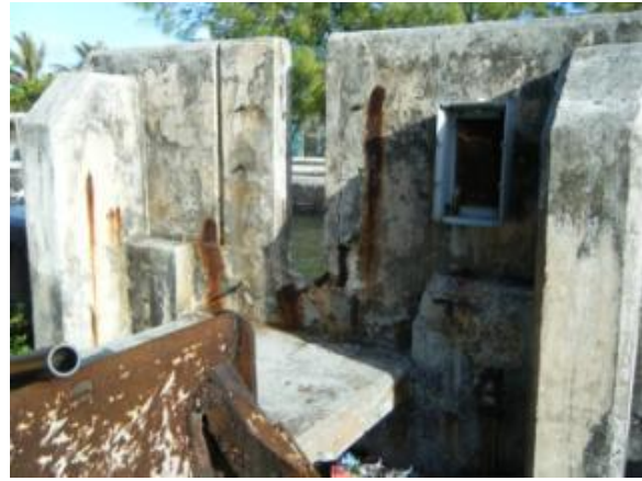
Figure 2.7 - Rotor seat empty and in need of repair
