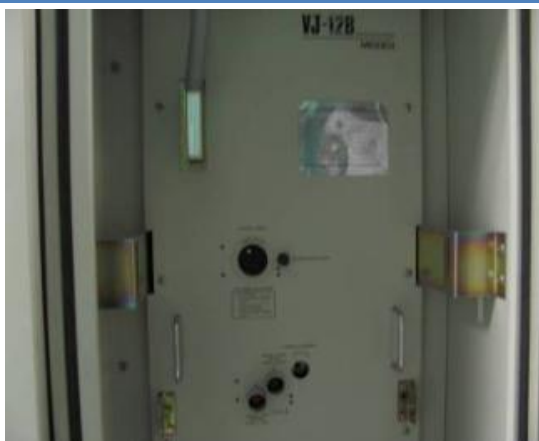
Figure 4.14 - Transformer Output Breaker
