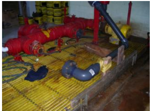
Figure 3.7 - Well Pump 2 (North)
