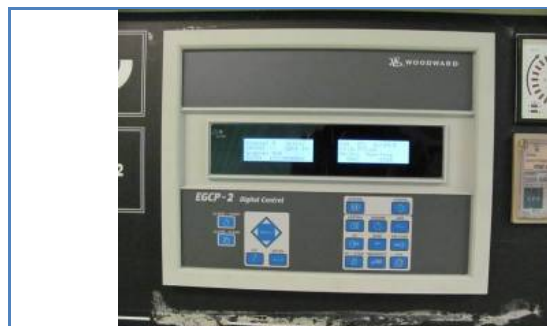
Figure 4.7 - Typical Generator Relay Panel
