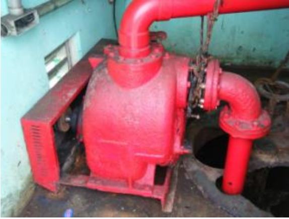
Figure 2.10 - Lift station #3 is the only one with an original pump, but the backup is gone
