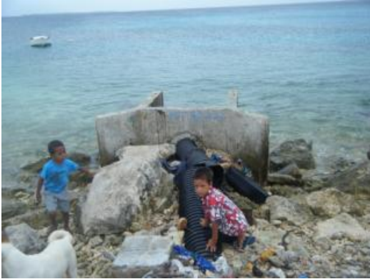
Figure 2.18 - Outfall exposed due to erosion and damaged
