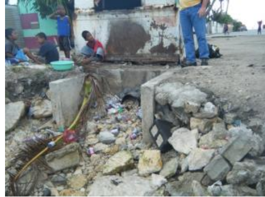
Figure 2.19 - Outfall clogged with sand
