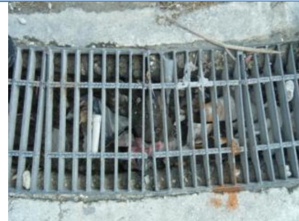
Figure 2.17 - Most trench drains were filled with either dirt or debris
